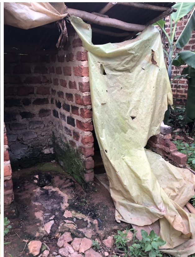
Non-Acceptable quality latrine
